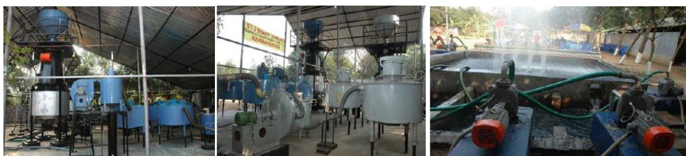
Figure 7, Rice Husk fired 250 kW Gasifier power plant and Spray pond at Kapasia, Bangladesh.
