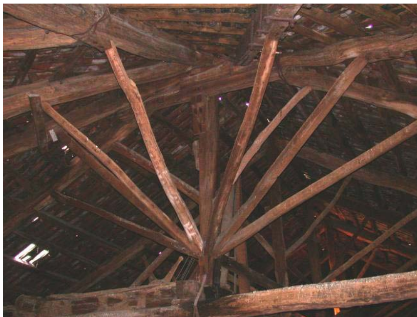
Figure 1 – Elements of the roof timber structure over the apse of the Cathedral of Vercelli Grading according to resistance
